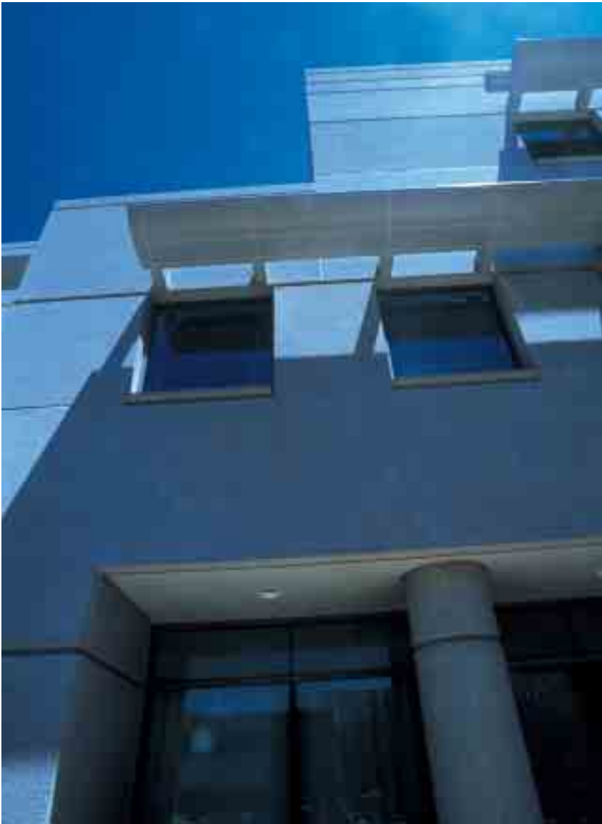
Aluminum sun shades were installed over each window to cut energy costs. The braces were set into the architectural precast panels, providing a slim profile that doesn't detract from the building's sleek lines.
